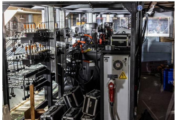
Below: 48-point plc motion control system
