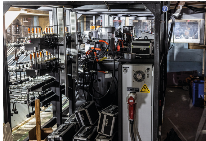
Below: 48-point plc motion control system
